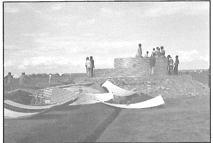
Construction of an OXFAM tank with semi-skilled refugee labourers Photograph by Robert Hodgson
