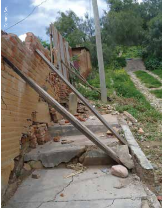
Walls propped up, post-landslide, Cochabamba.
