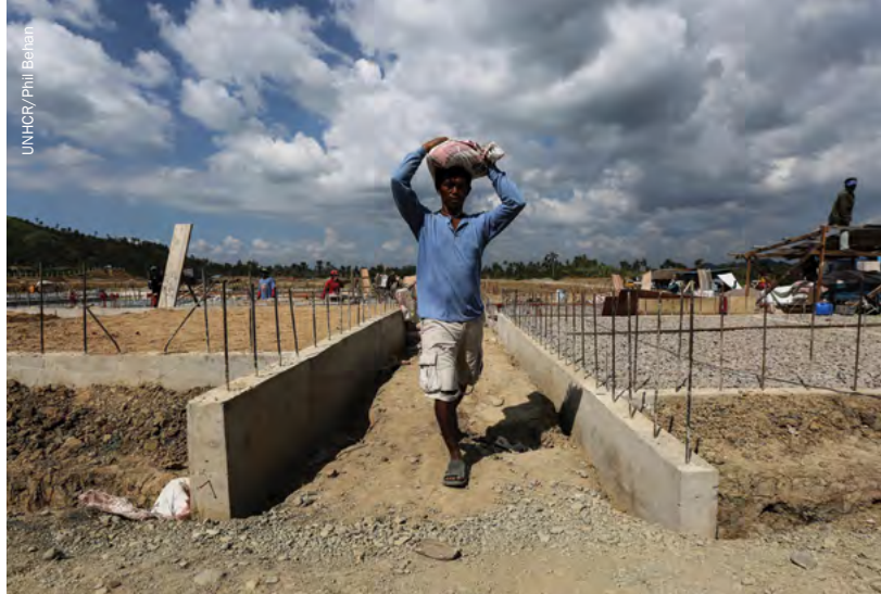
Joel Lacaba working on the construction site for his future permanent home in Tacloban, part of a recovery programme after Typhoon Haiyan, the Philippines.
