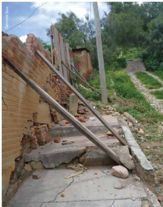
Walls propped up, post-landslide, Cochabamba.
