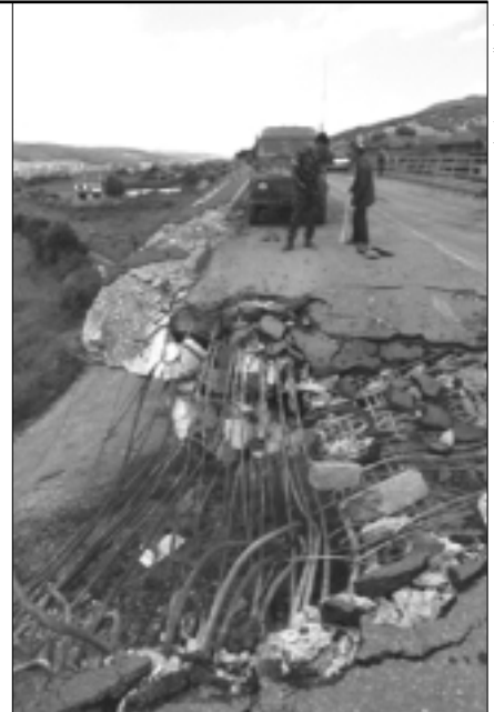
Bomb damage to road bridge between Pristina and Podujevo
