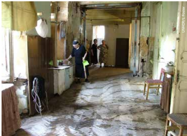
Originally a hospital until condemned as unfit, this building in Tbilisi, Georgia, was re-opened in 1993 to accommodate IDPs from Abkhazia.
